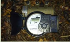
How the Meter Should Look in the Box
